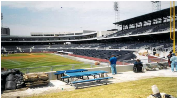
ECI provided technical assistance on ADA accessibility requirements for Harbor Park Baseball Stadium
